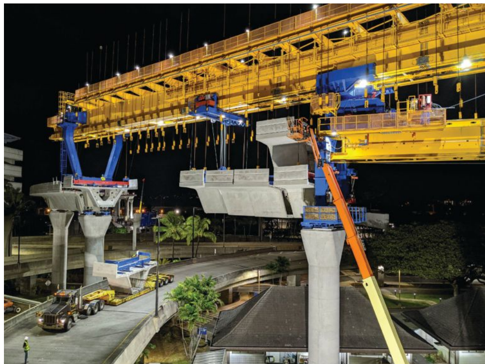
Figure 4. Nighttime installation of precast concrete segments within the footprint of Daniel K. Inouye International Airport. More than 2700 segments were cast at a nearby facility and transported approximately 20 miles to the jobsite. Photo: Shimmick, Traylor, and Granite Joint Venture.
