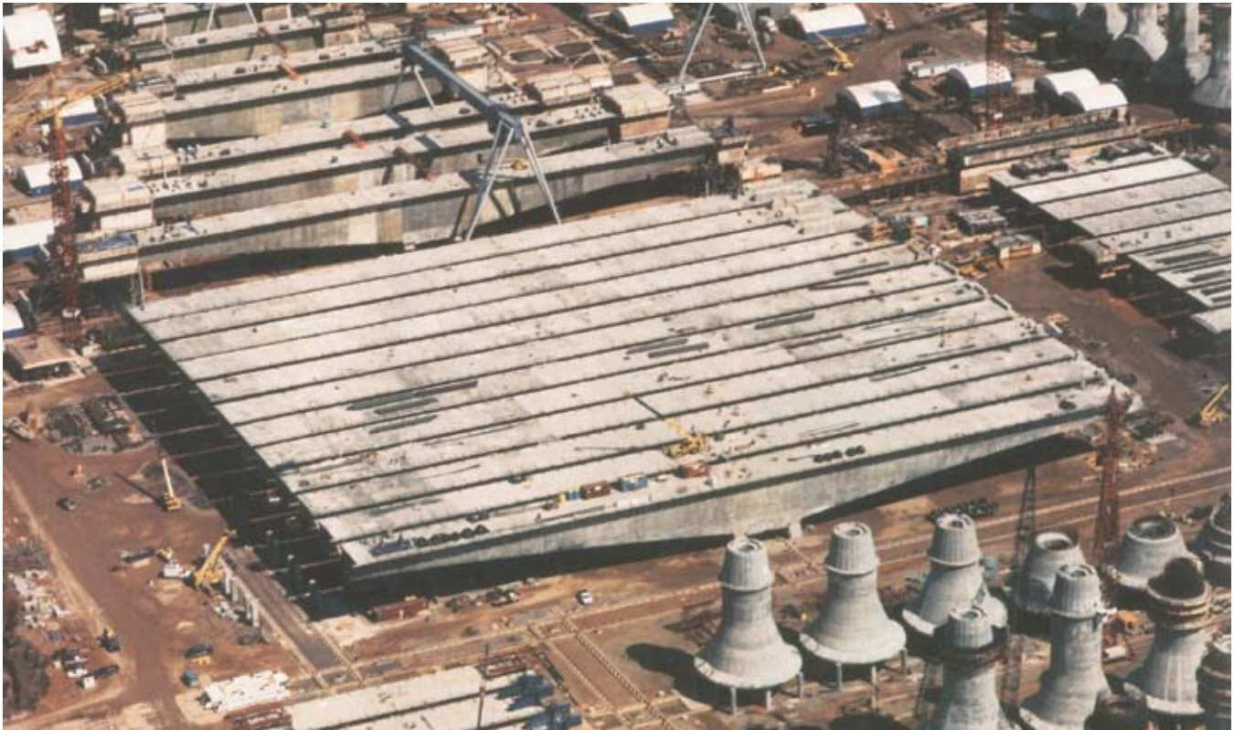
Fig. 26. Shown is the Confederation Bridge precasting yard in Prince Edward Island, Canada.
