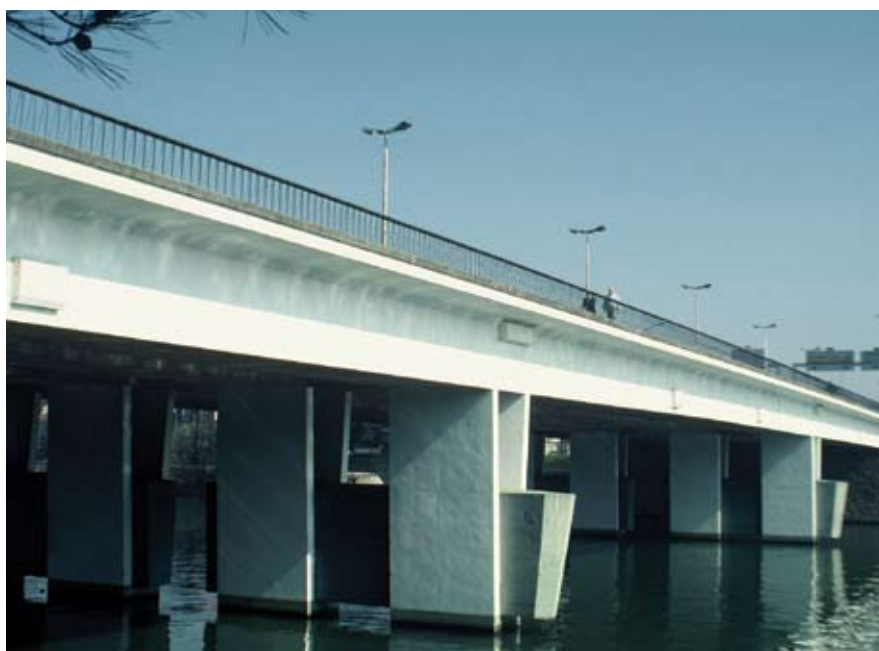
Fig. 6. Shown is the Choisy-le-Roi Bridge over the Seine River in Paris, France.
