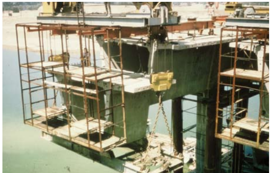
Fig. 9. Shown is the Pierre Benite Bridge over the Rhone River near Lyon, France.
