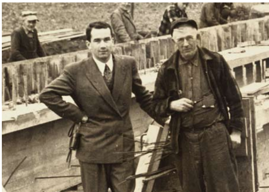
Fig. 5. Jean Muller (left) is photographed at the Shelton Bridge site in upstate New York.
